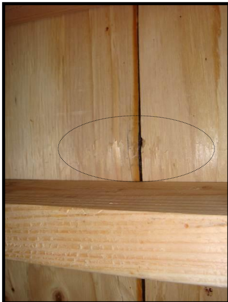
Figure 4a. Buckled Plywood Shear Perpendicular to Rafter
