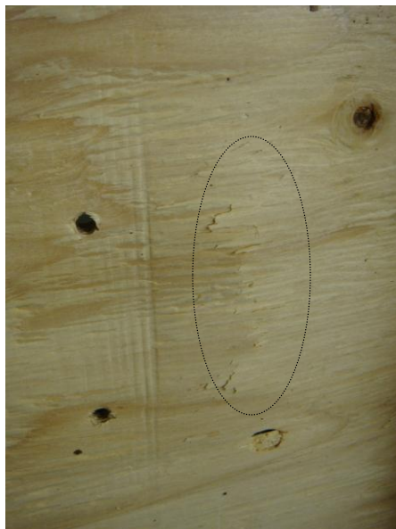
Figure 4. Buckled Plywood Shear Perpendicular to Rafter
