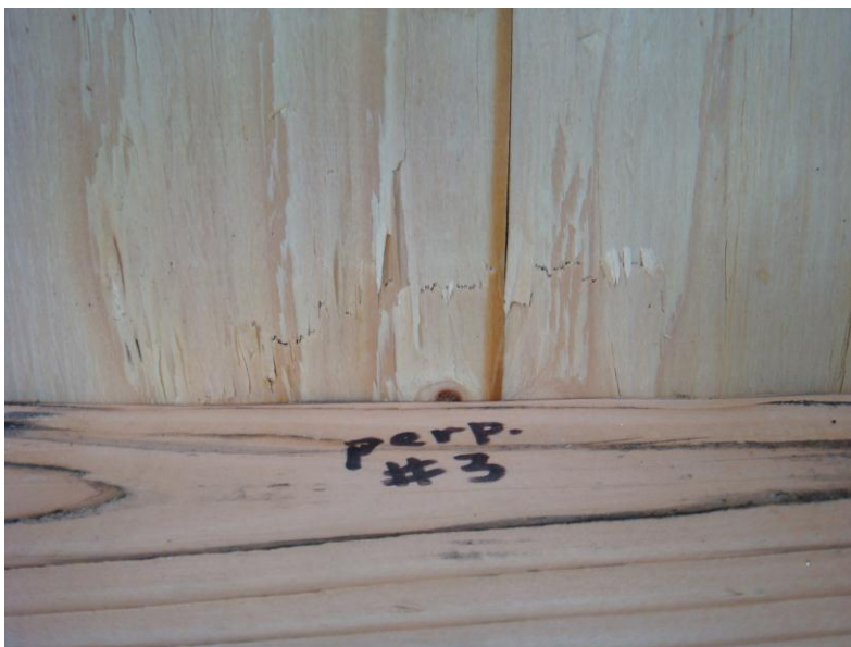
Figure 4. Buckled Plywood Shear Perpendicular to Rafter
